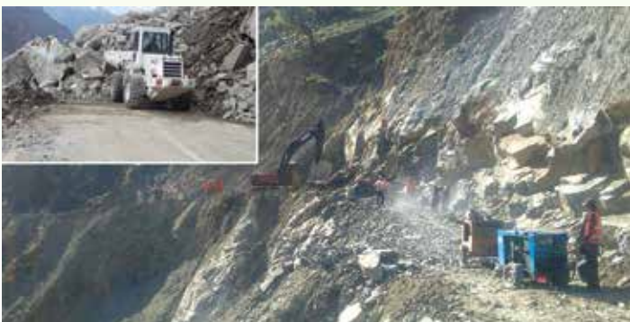
Gilgit Baltistan 15 April 2016: Efforts for clearance of landslides
